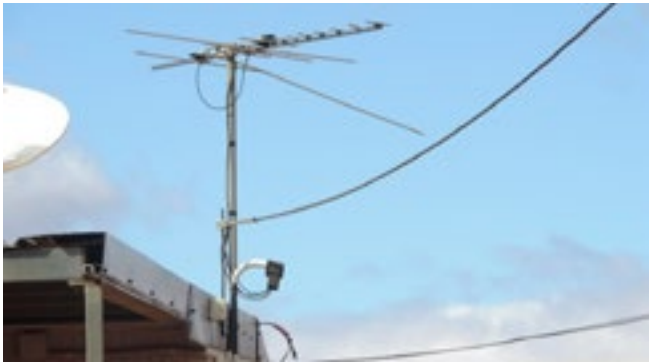
Image: PVC service wire and twisty replacement
